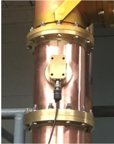
Indoor Sensor installed at the transmitter output
