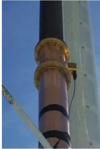
Outdoor Sensor installed at the top of the tower
